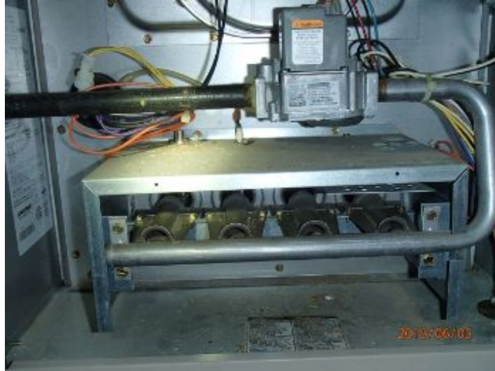
HVAC equipment should be serviced at least once each year
