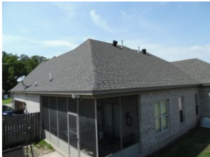
Turbine vent is damaged
