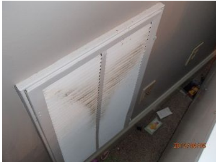
Return air grilles in all bedrooms. Change filters each 30 days
