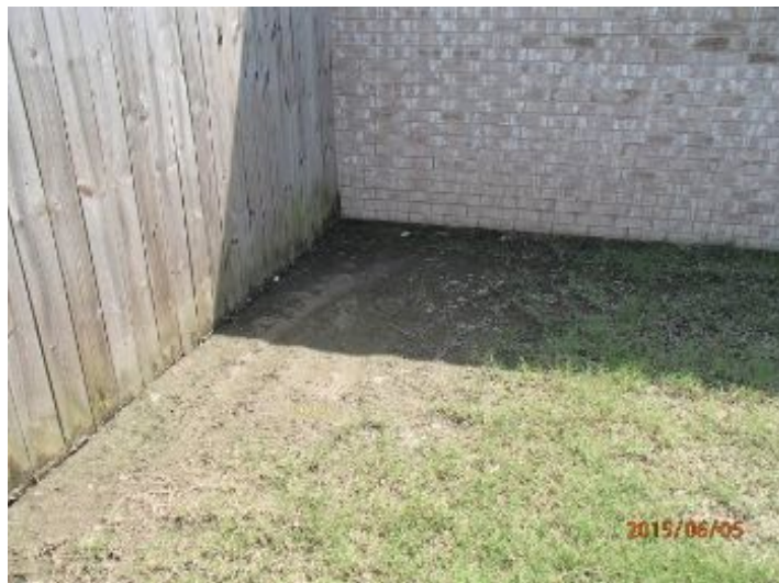
Poor drainage. French drain, regrading or other repairs needed
