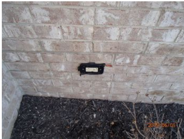
Damaged/missing receptacle cover near front entry
