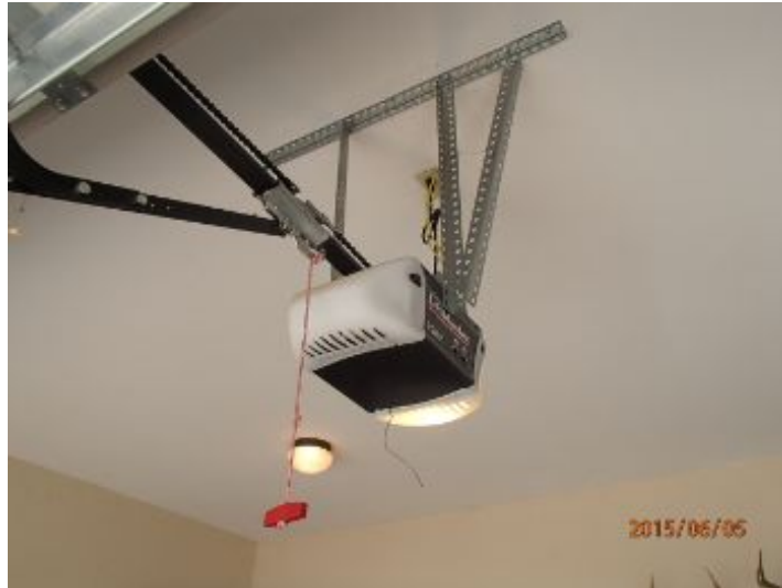
Functional. Adjustment needed to closing force of operator
