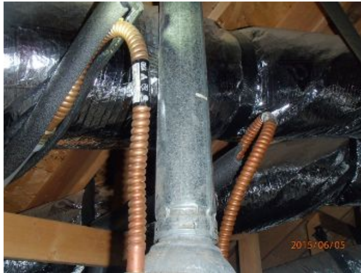
Flue pipe is to close to HVAC duct
