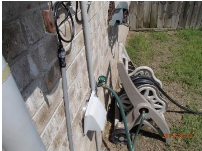
Dryer vent loose at wall
